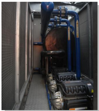
Internal view of the rental unit showing the compressors and flooded evaporator
