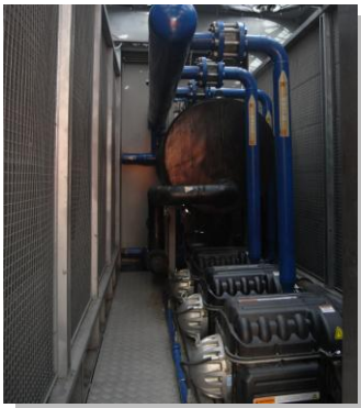
Internal view of the rental unit showing the compressors and flooded evaporator
