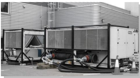
The modified Modular SRAT chiller installed providing emergency process cooling
