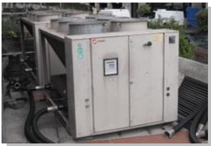
Trane emergency chiller hire system, serving building air conditioning and computer rooms
