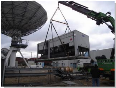
The Carrier 30 GX rental chillers being lifted into position by Hiab lorry
