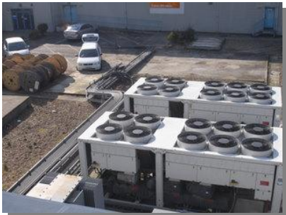
The completed rental installation providing data centre chilled water for close control units
